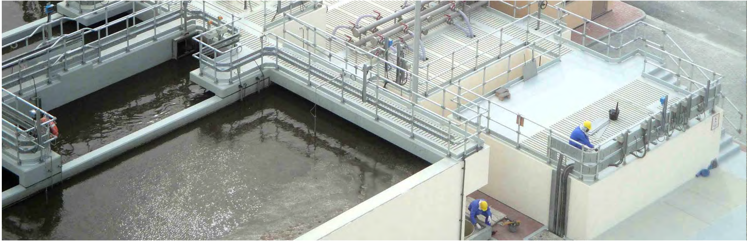
Ma'Amir & North Refinery Industrial Area Sewage Treatment Plant
